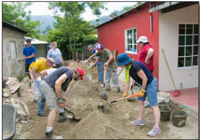
Christ Church (Valdosta) Missioners mixing concrete in the street to pour a floor for the house we built this year for our translator and friend Leidy Rosario and her family in El Pedregal near Jarabacoa.
