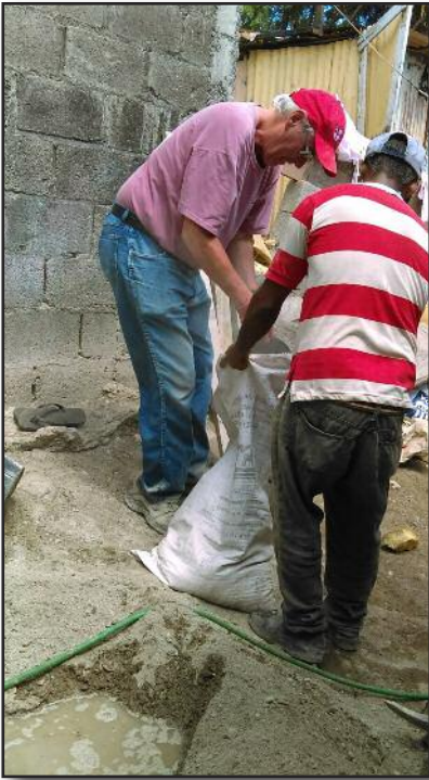
St. Anne's (Tifton) pouring concrete to build bathrooms in the village of Las Carreras.
