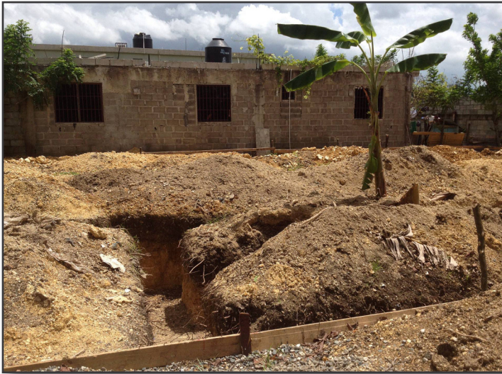
Preparing the foundations for Iglesia Episcopal San Pablo y San Lucas in San Isidro.
