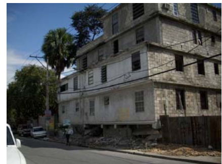
Pancaked building down onto first floor
